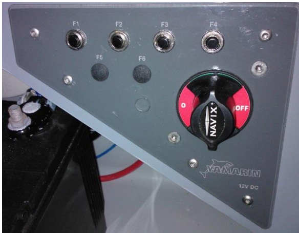
Main power switch and circuit breakers.
